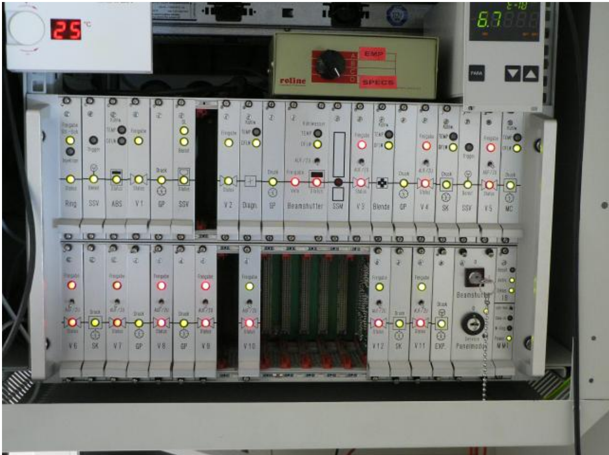
Figure 1: beam valve control panel with "roline" control box (to switch between XPS and NEXAFS); in the upper right corner you see the pressure reading of the beamline part just behind valve 13 on the beamline side.
